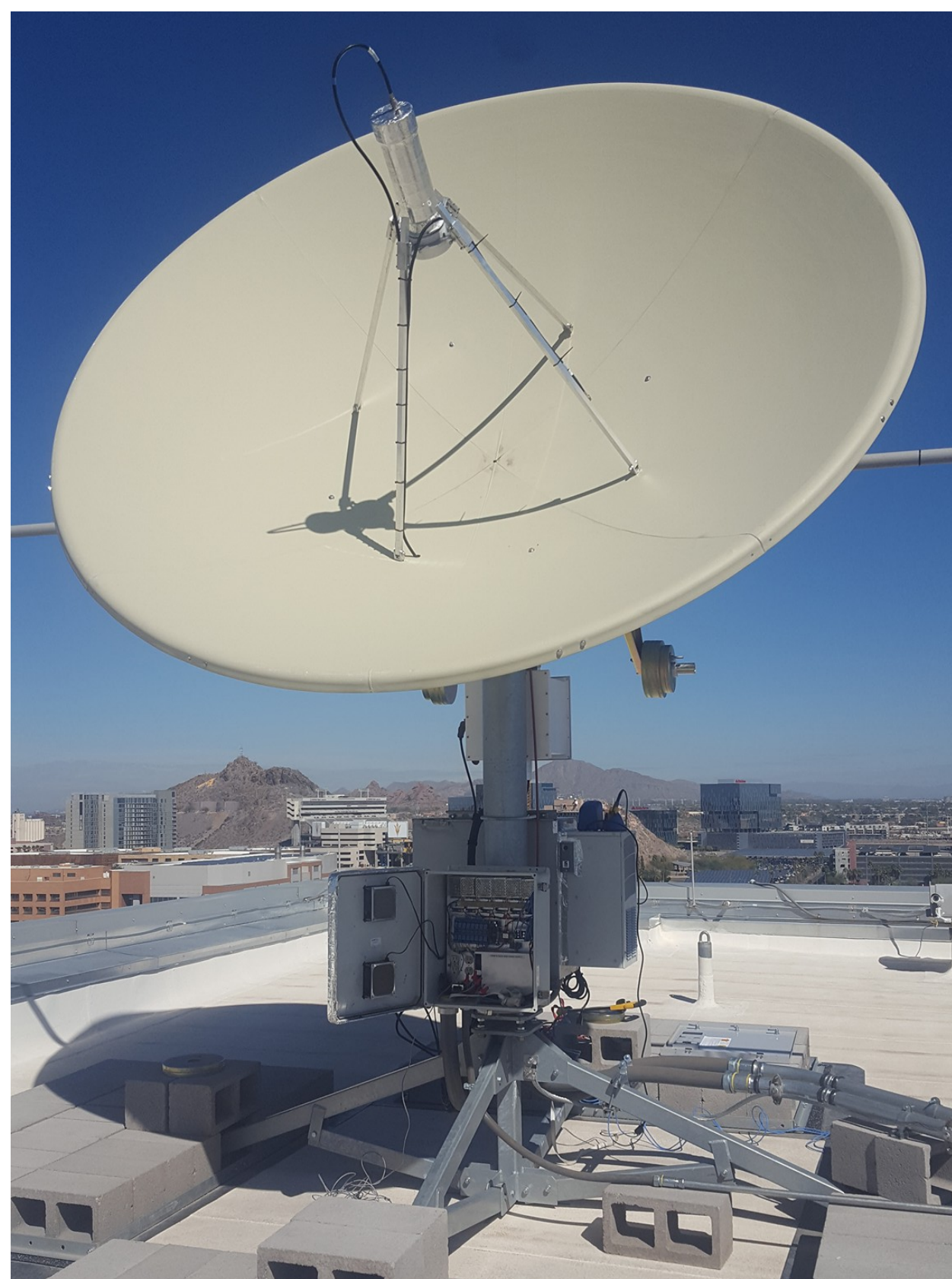
Figure 2: Installation of revised ground station on the roof of an ASU building in February of 2018. Replaced parts include a steel-case rotor, 75% lighter dish. Upgrades include a new student-built power control box, and a weather station.
