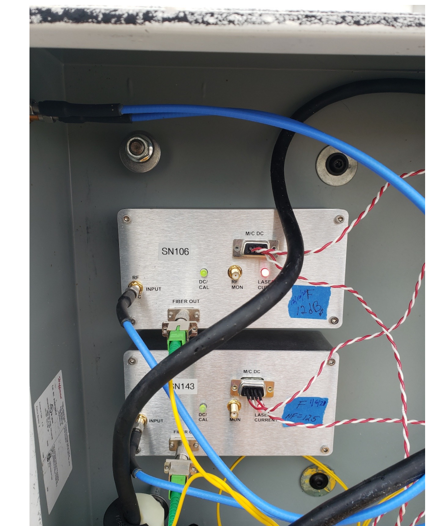
Figure 3. New FEBs installed at Delta CRABS station.
