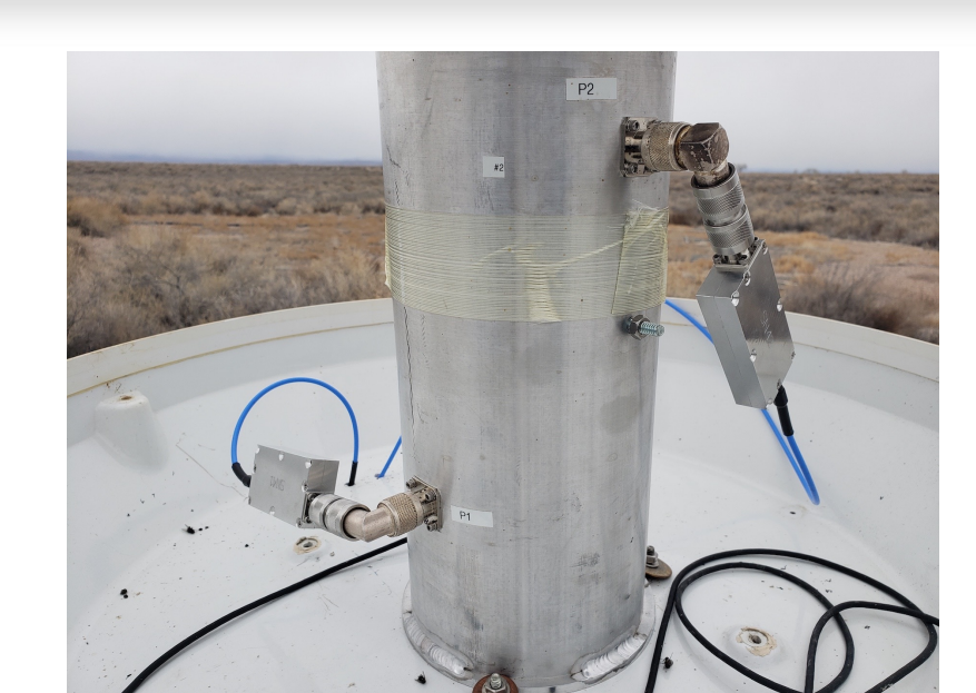
Figure 2. Upgraded LNAs installed at Delta CRABS station.
